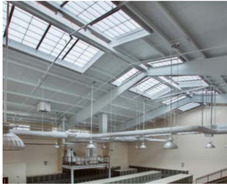
FY14 TEMF COF — Joint Base Lewis McChord, WA, US Army Corp of Engineers-Seattle Div., Guardian 275® Skylights
