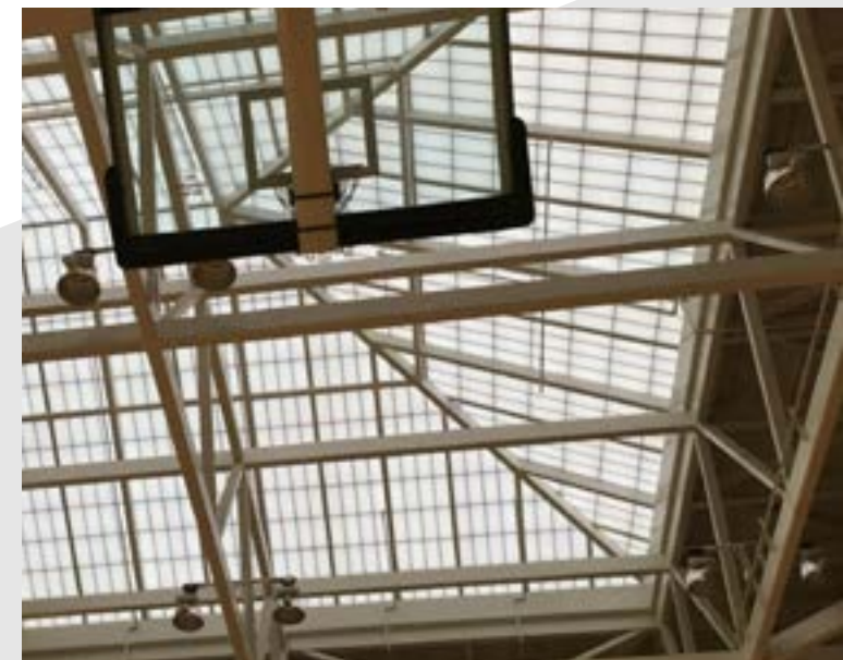
Above: U. of Georgia Ramsey Center Skylight Replacement — Athens, GA, Guardian 275® Hip Ridge Skylight
