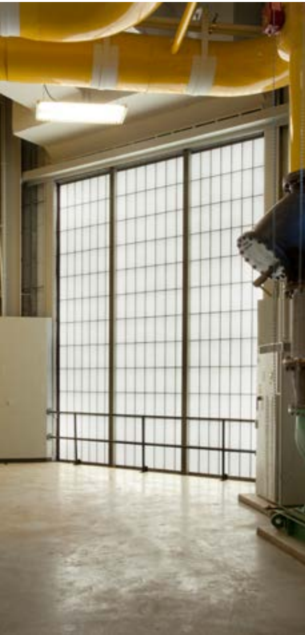
BSU Geothermal Plant – Muncie, IN., MSKTD & Associates, Inc., Guardian 275® Wall System
